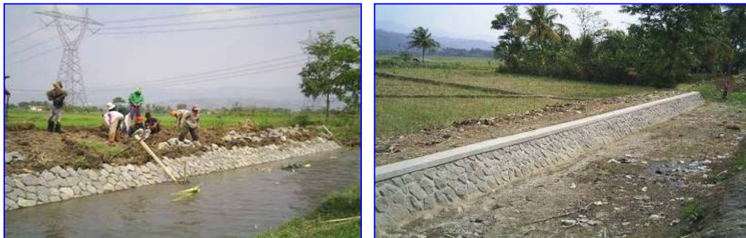
Step VII. Illustration of the finalization of mutual work activities of maintenance works, canal improvement and other physical activities of irrigation O&M.
