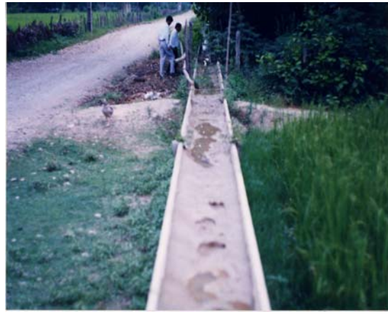
Photograph 3. Obstruction Created by Accumulated Sediments and Growing Plant in the Canals
