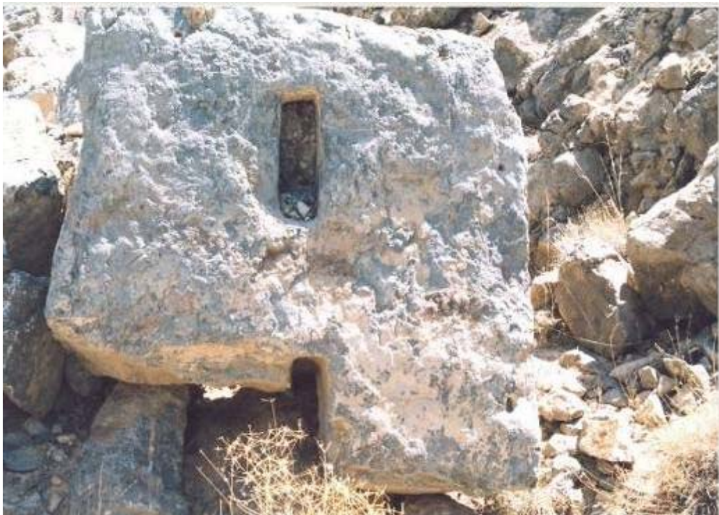
Figure 17. Bottom of a piece of UU-shape stone with slots for fixing wooden slide gates in them. This has been an element of a water conveying system downstream of Didegan storage dam.
