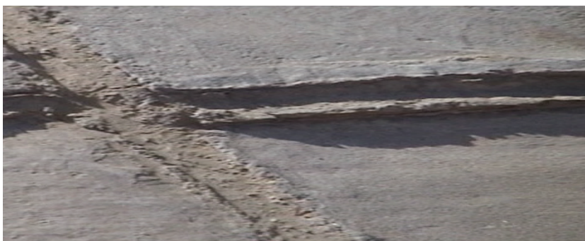
Fig. 3. the concrete lining destroyed by freezing-thawing and frost-heaving
