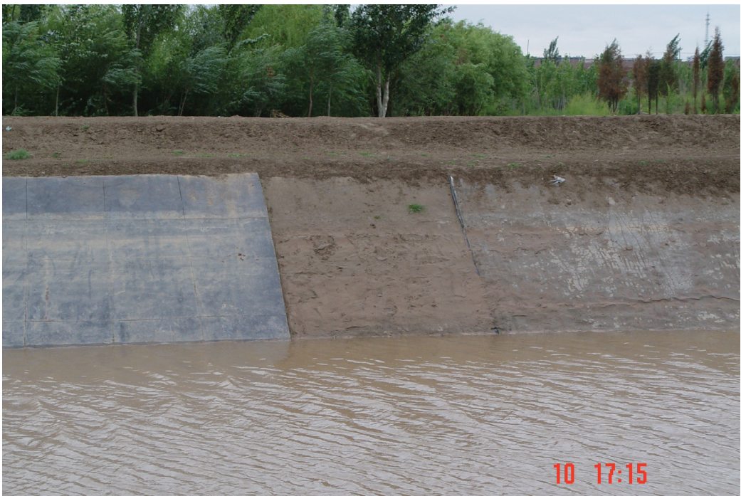
Fig. 5. the stability of side slopes applied with GCL in Yonggang sub-main (treatment of nature soil covered)
