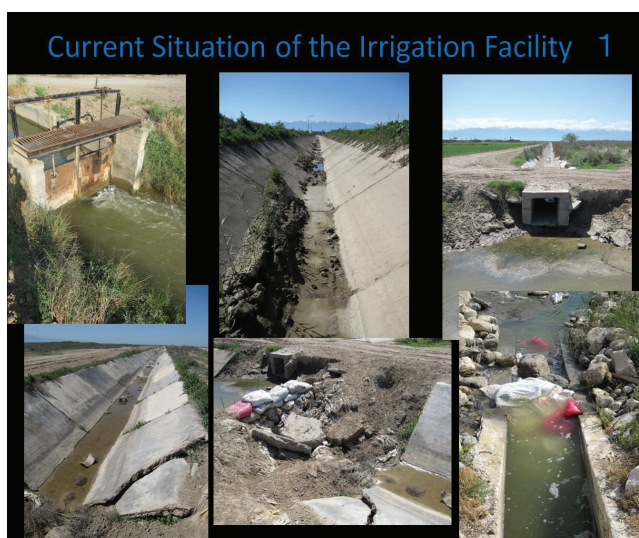
Fig. 3. Current Situation of the Irrigation Facility
