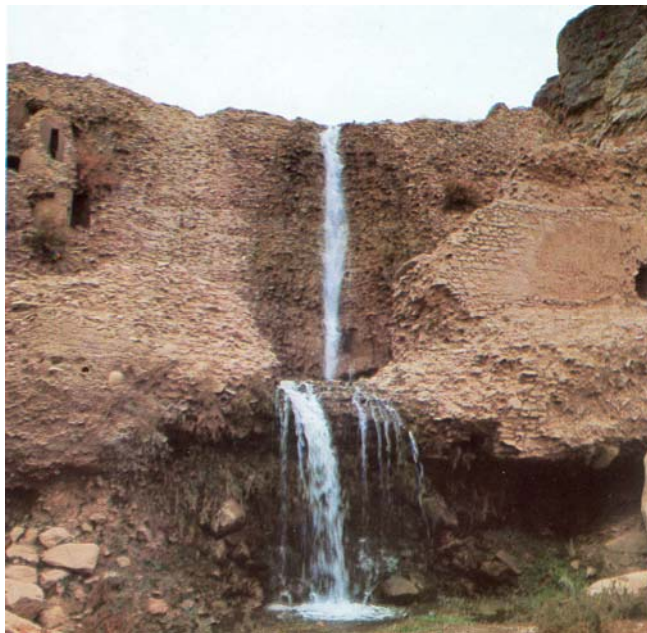
Fig 100 , Qamsar Weir, the reservoir is filled with sediment and the body was ruined. The picture shows the quality of lime concrete, there is water tower in the middle with stairs made of bricks.
