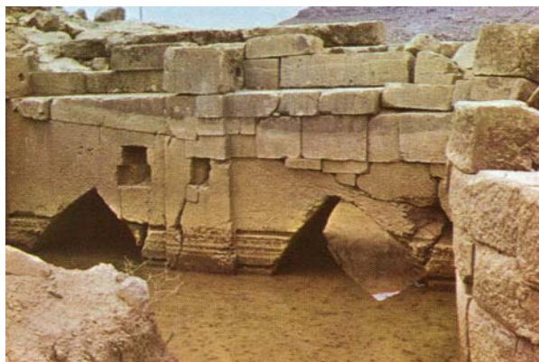
Fig 50, The remains of water intake from Darius The Great Weir on Kor River
