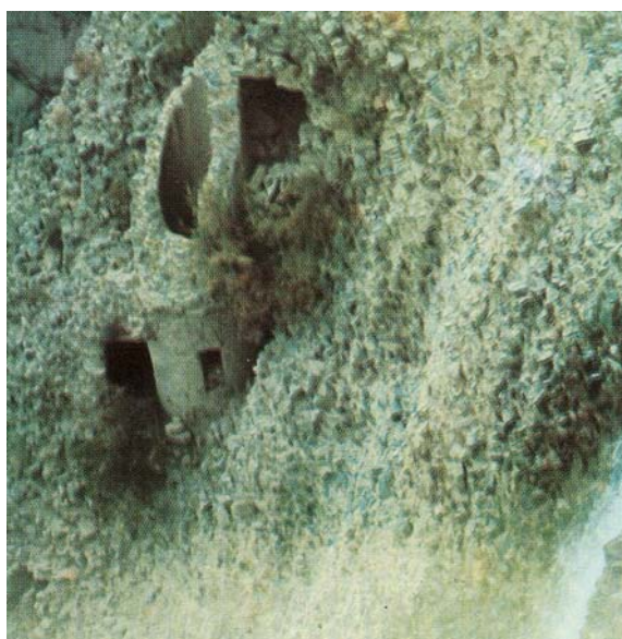
Fig 80 , Qamsar Weir, view from downstream. It is possible to see the lime concrete of the body in the middle. There are the remains of one of the water towers.
