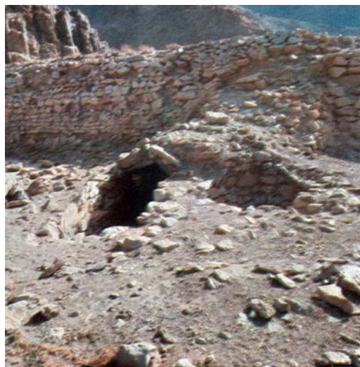
Fig 78 , Qohrod Weir in Kashan, view from upstream. The reservoir is full of sediment. Water tower can be seen in front
